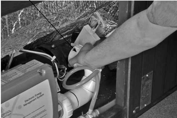
RELEASING AN AIR LOCK...
